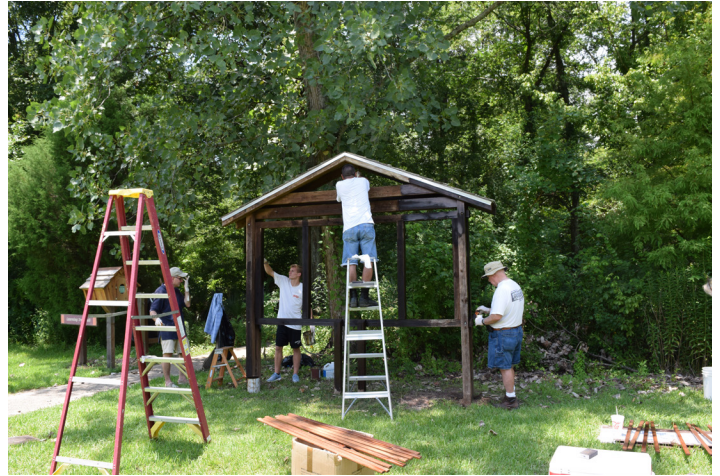
Congratulations to Graham Frazier who earned his Eagle Scout badge through organizing the renovation of the trailhead kiosk and adding the Burden Woods trails to the AllTrails app. Graham is pictured second from left. Other helpers with the project included: Deane Frazier, Scott Frazier, Jimmy Giroir, Aaron Tucker and Brant Mangum.
