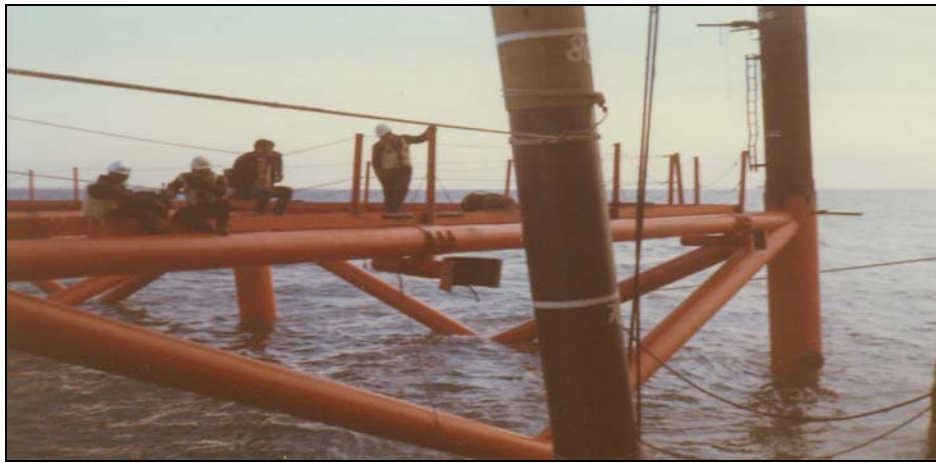
Figure 6.3. Preparing to Remove a Jacket Leg from a Platform Skeleton. Photo Courtesy of Joseph Schouest, OOGHP.
